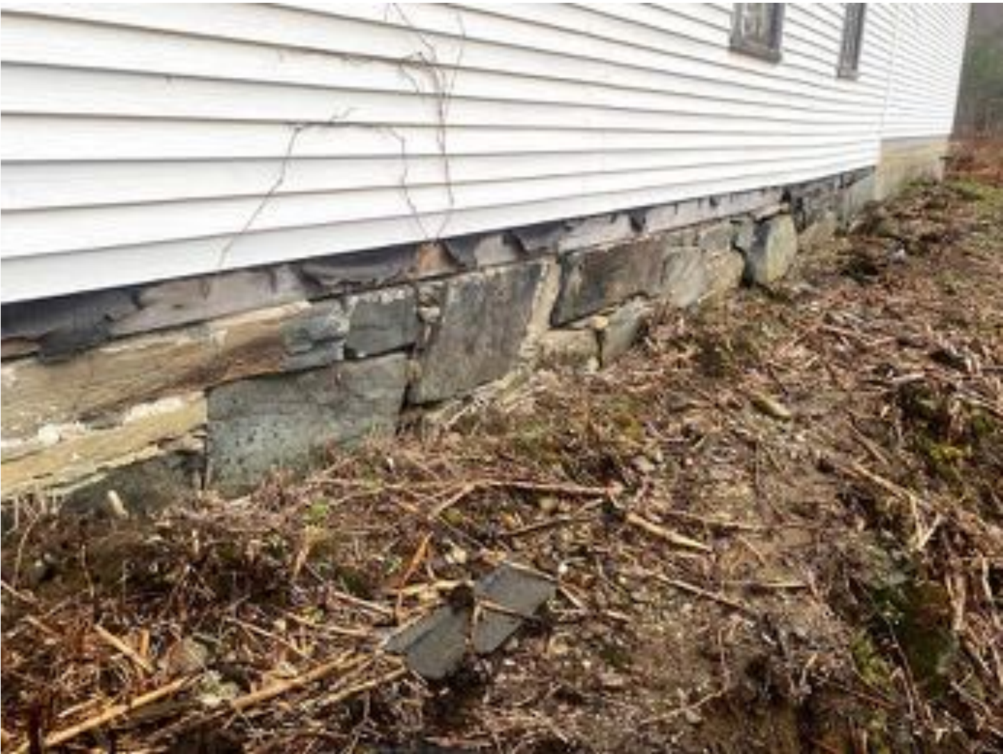
The stone foundation on the North wall. A few of the stones have shifted and need to be reset but the majority of the stonework simply needs repointing. The original mortar was lime-based and replacement mortar should be mixed to match the original.
