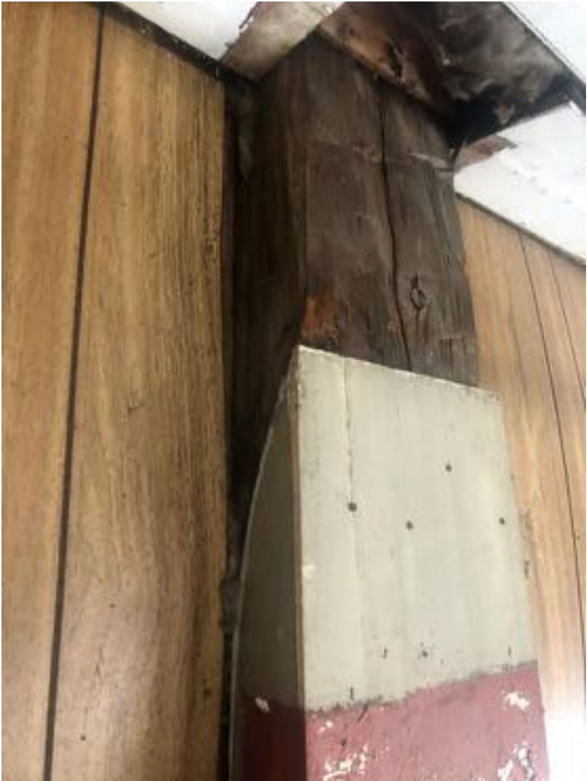
Post casing, showing the steep coved ceiling that was likely original to the church. Removal of the newer beadboard ceiling should uncover the top of this curve.
