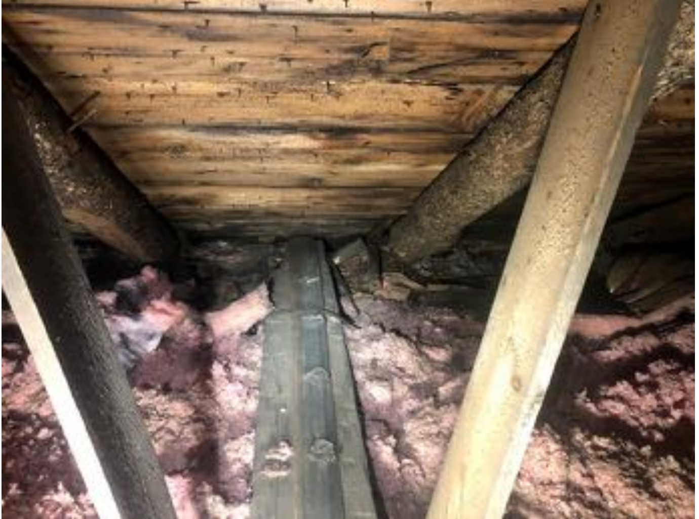
Cutting edge from a plow attached to the top of tie beam three on the South end for reinforcement.
