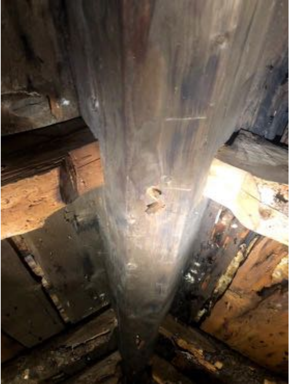
Close up of the five-sided ridge and rafters. It appears that the geometry of the hewing is off slightly with the South side being slightly steeper than a square angle to the roof, which is the typical design. This is likely an error in the layout of the hewing .
