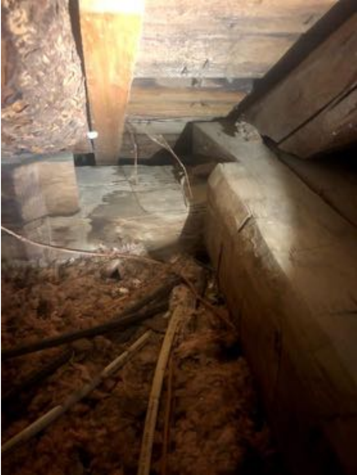
The connection from tie beam to plate in the Northeast corner. The top plate has a half lap much larger than the width of the tie beam on both the North and South ends of the first bent. This is a peculiar detail, along with the rafter spacing, and suggests possible re-use of the plates as well, or simply a mistake in the joinery.
