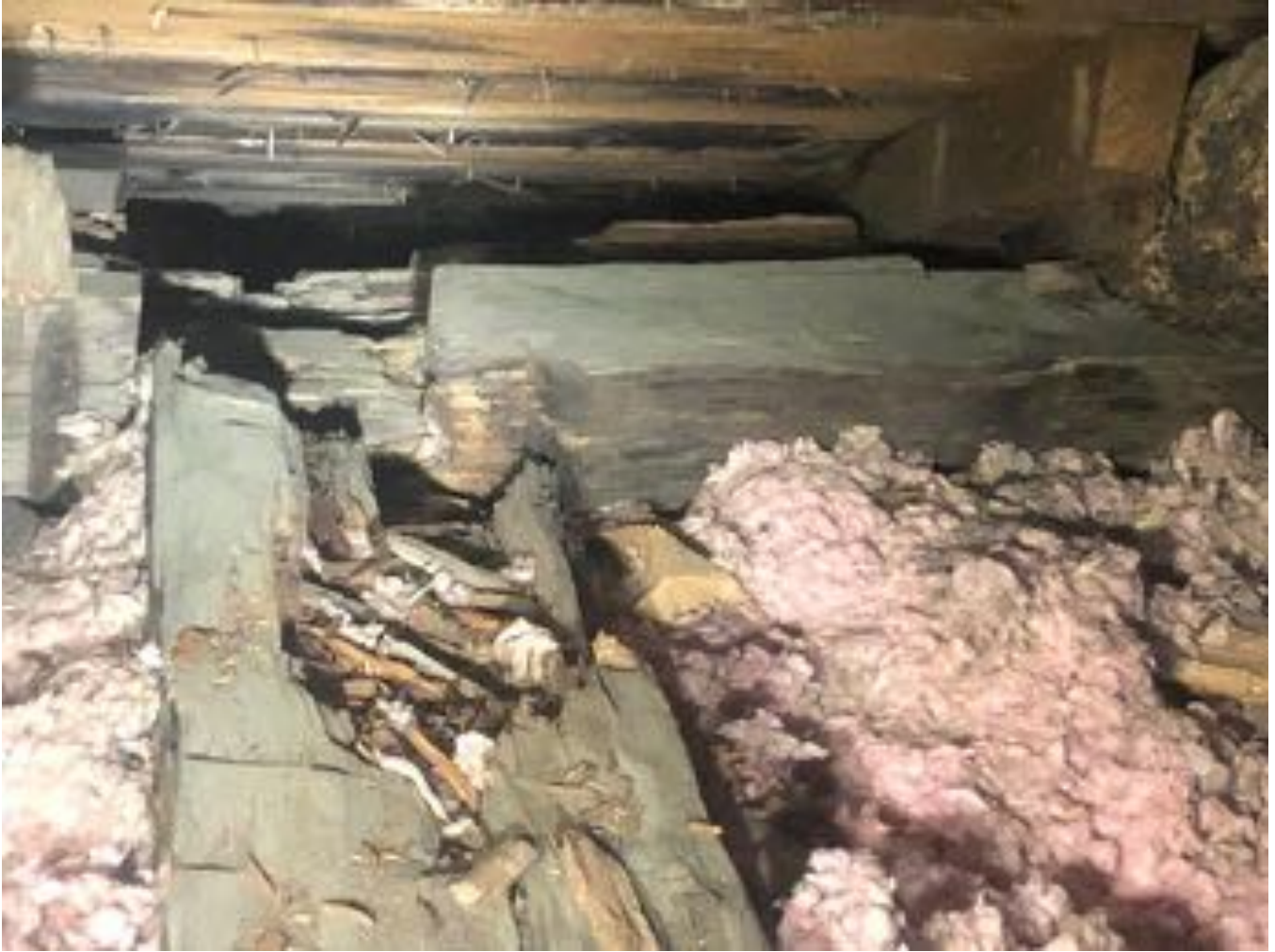
Severe rot at the South end of tie beam five.
