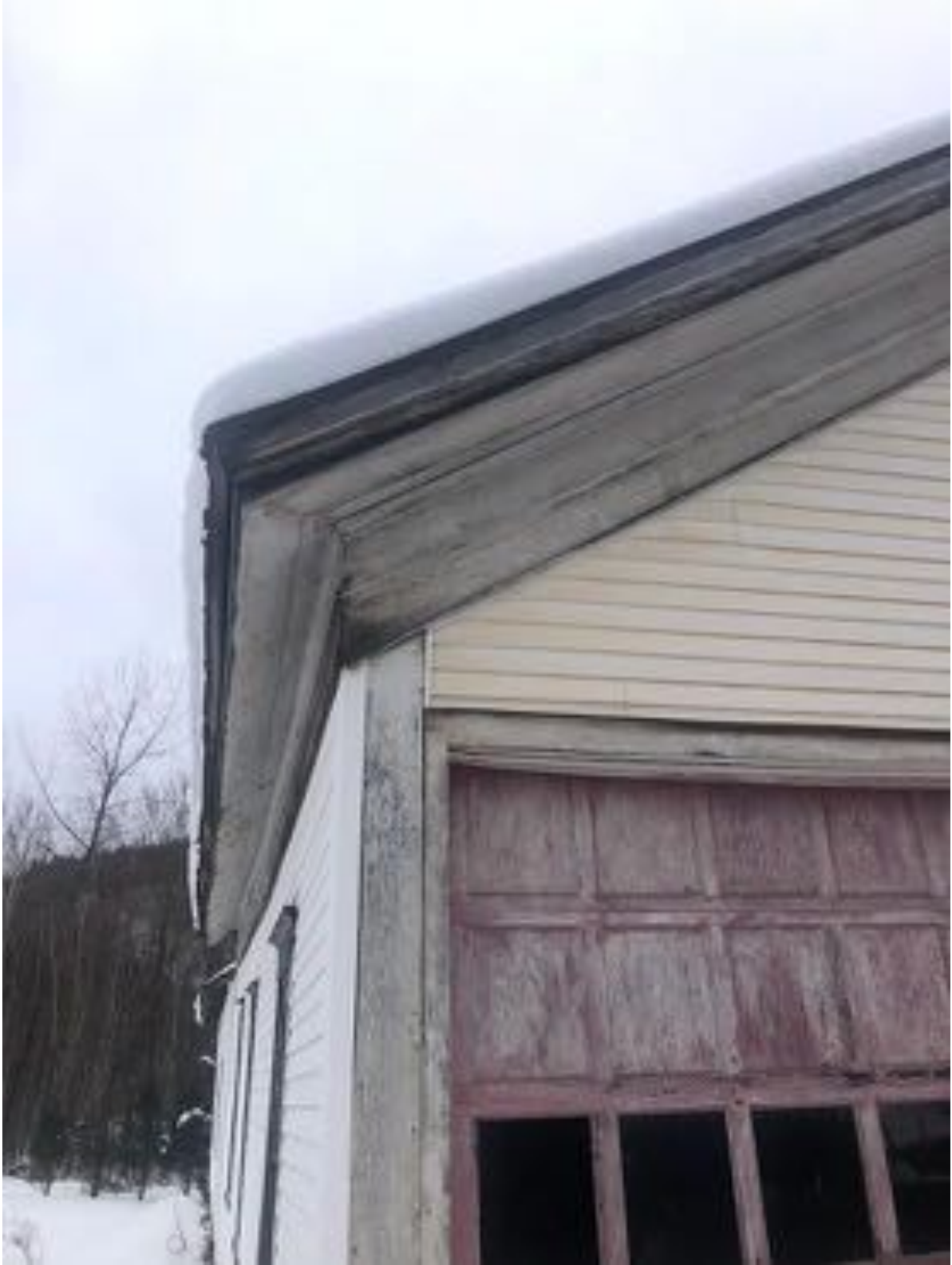
The Southeast corner roof trim detail, with a double frieze and deep soffit, adding to the simple vernacular elegance of the original building.
