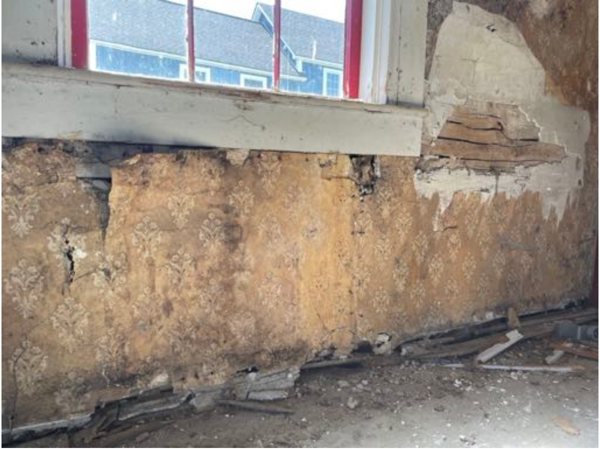
Split lathe and plaster, covered by wallpaper . The window trim and portions of the baseboard are still intact.
