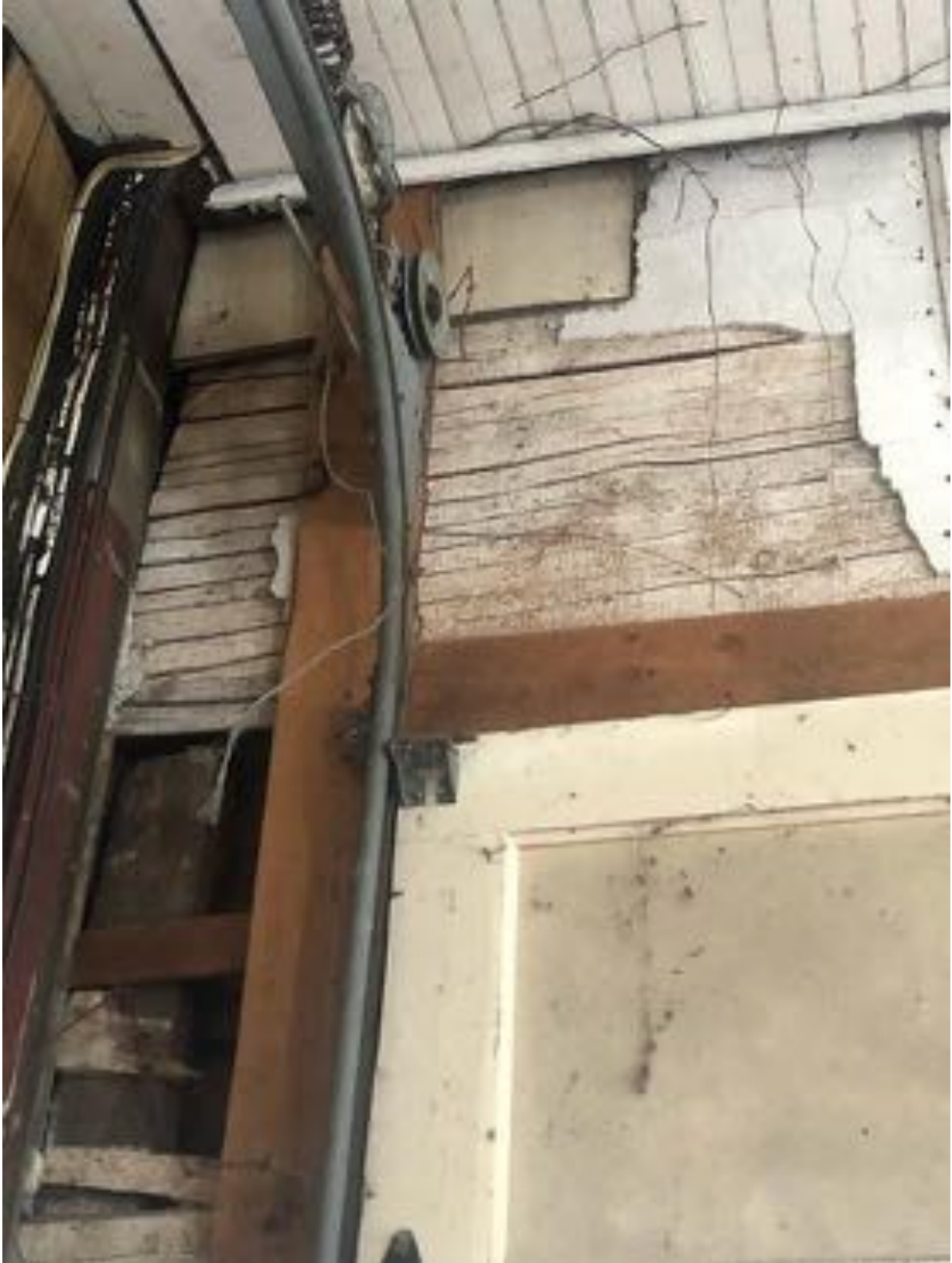
A small section of split lathe and plaster that was uncovered behind the 1980's paneling. Cut lathe replaced split lathe around 1850, so this section of wall predates that transition and is likely original to the structure.
