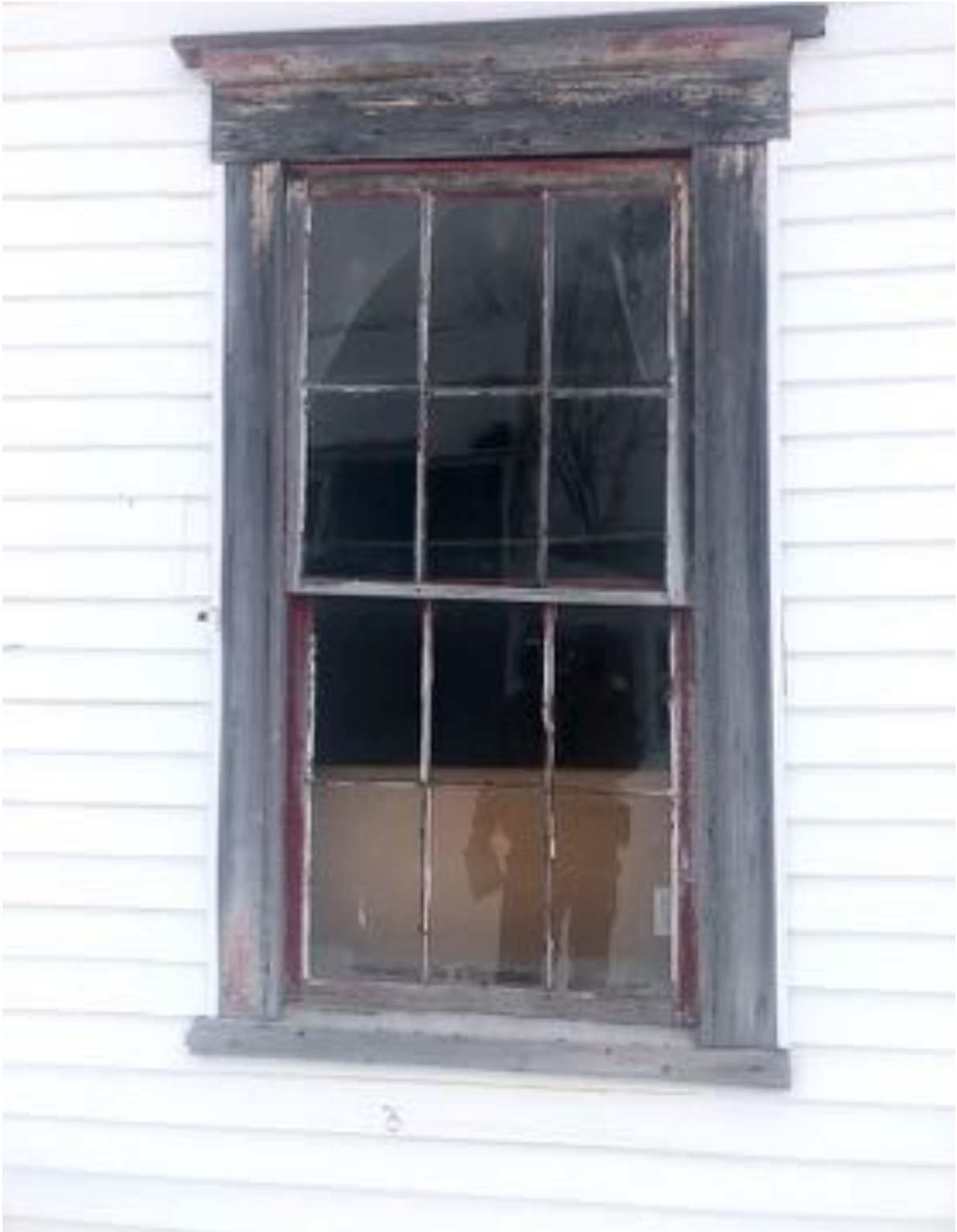
Six over six window on the North side of the building with the original trim and vinyl siding added. The existing woodwork is generally in good condition throughout and generally only in need of a thorough scraping and painting. Care should be taken to use precautions for lead in the paint removal process.
