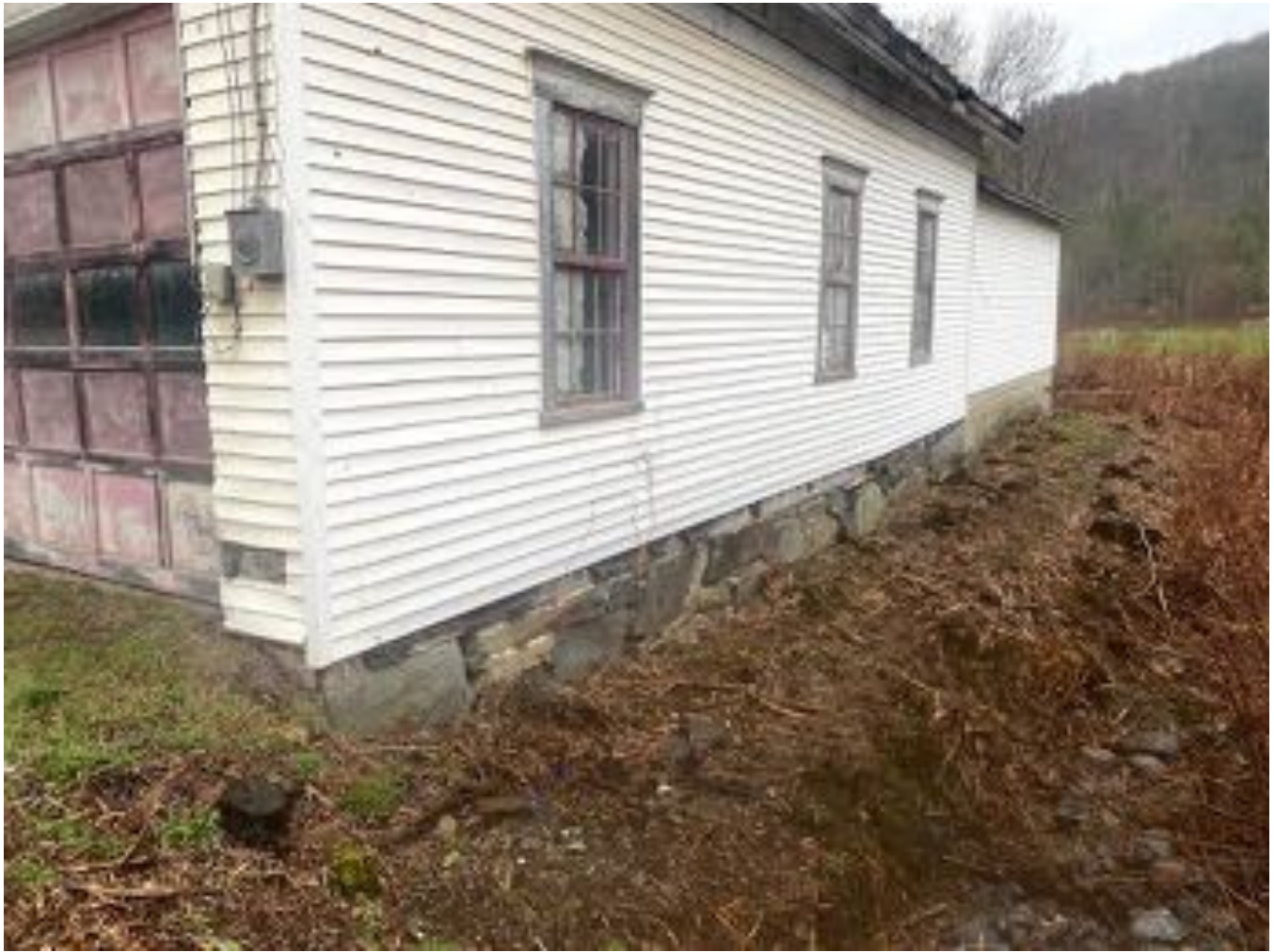
The North side of the building, with the only portion of the stone foundation still visible. To the North of the building is a small drainage stream. The banks of this stream are covered in Japanese Knotweed, which is currently being managed.
